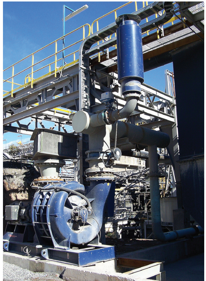
Three Power Mizer Series 7000 blowers are installed in a gold mining operation in Chile.
